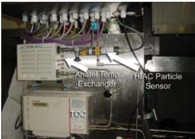
Figure 3. Instrumentation panel with HIAC HRLD sensor.
